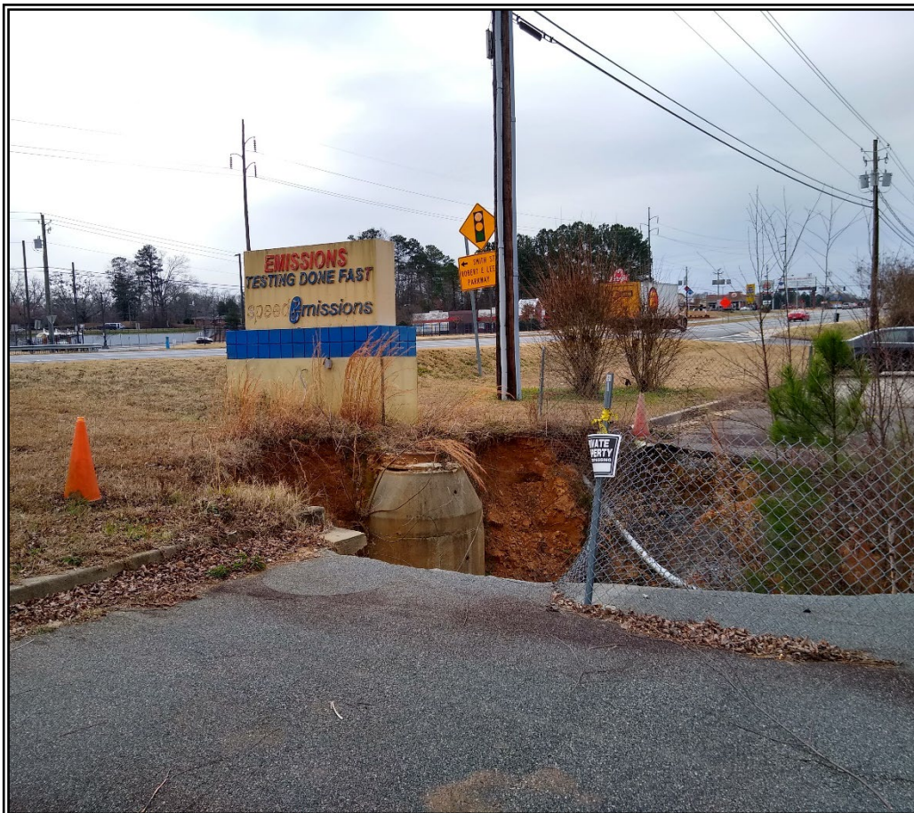
View of sinkhole around manhole, facing Tara Blvd.
