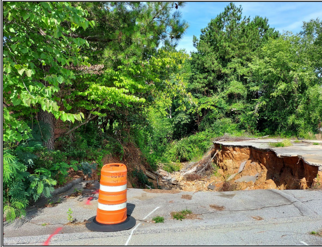
View of sinkhole, facing west.
