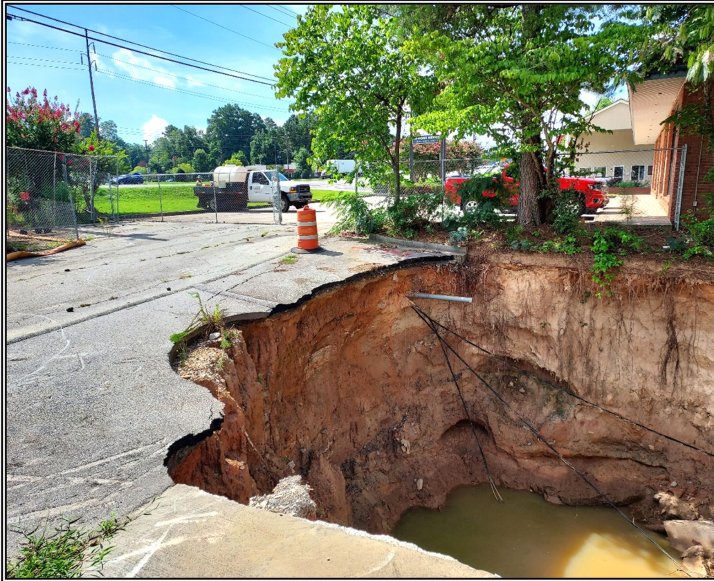
View of sinkhole and B1/B2 area.
