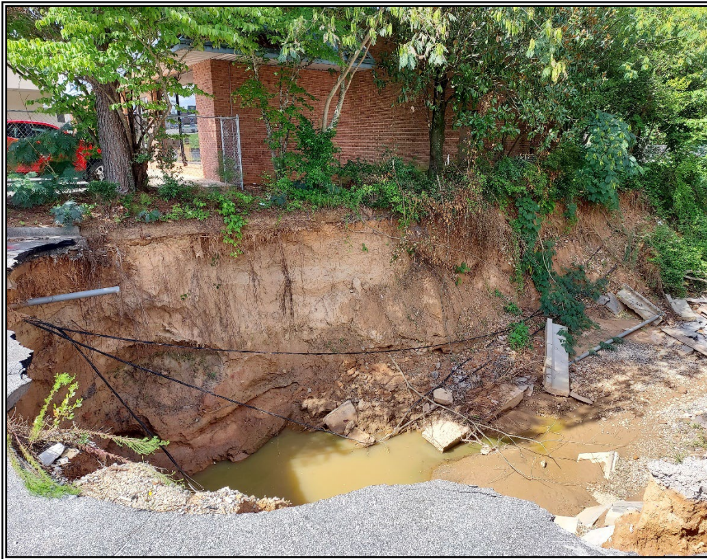
View of sinkhole and Leslie's Pool Supplies building.
