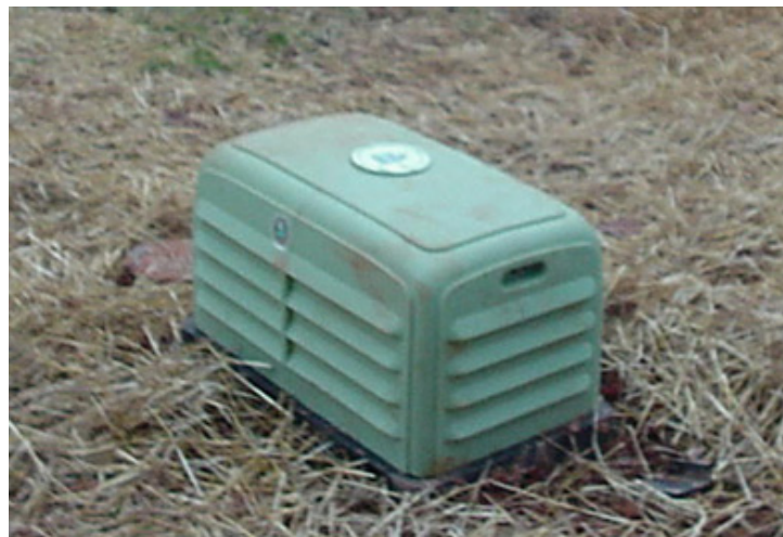
Clayton County Water Authority Automatic Water Distribution System Flushing Devices August 2006
